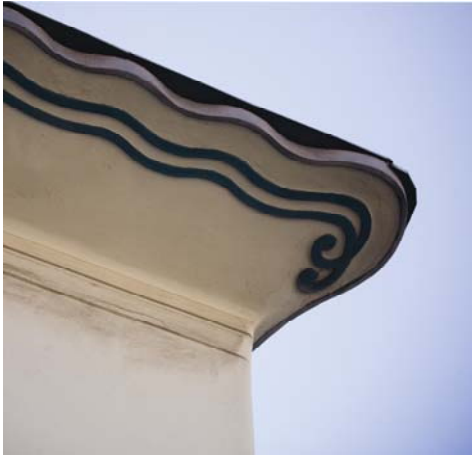
2.Szilard Zielinski, ex hotel Emigranti, detail of roof cornice (Photo Željko Stojanović)
